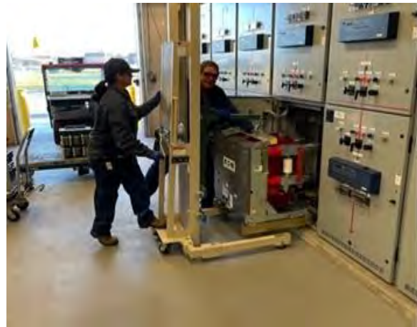
RWHTF and NTP maintenance staff working on NTP's breakers
