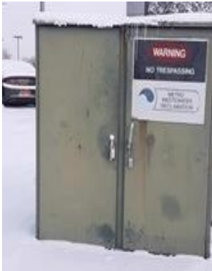
Typical Annual Charge Sampling and Metering Cabinet
