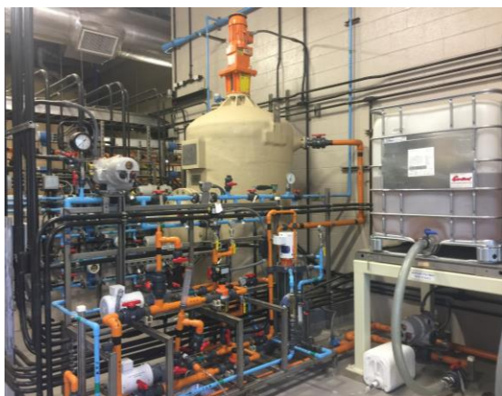
Tertiary Chemical Feed System
