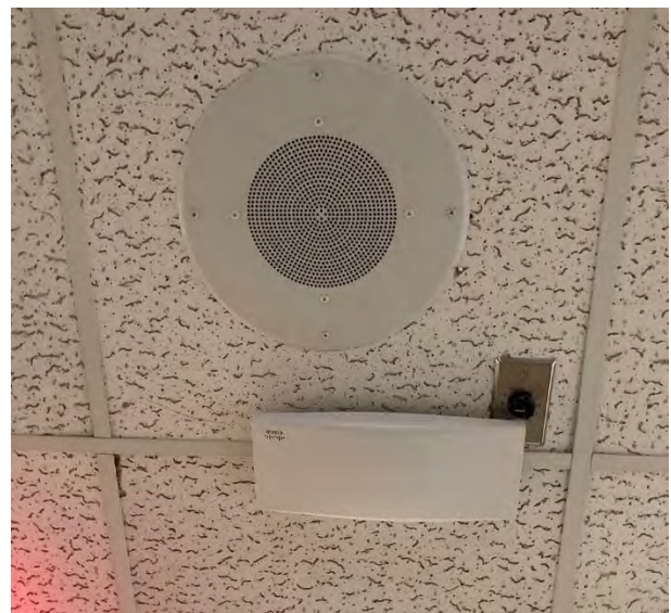
Example of an indoor wireless access point.
