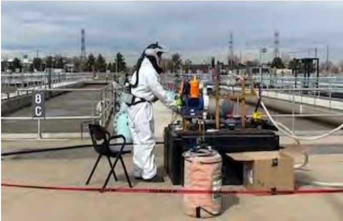
Rubyn McMaster monitors the acid injection pump.
