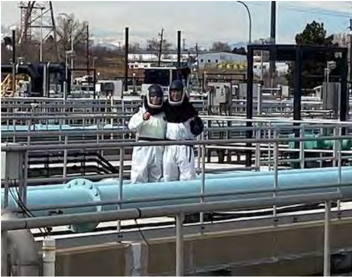
David Usher and Alex Martinez moving hoses and inspecting connection points to avoid any leaks.
