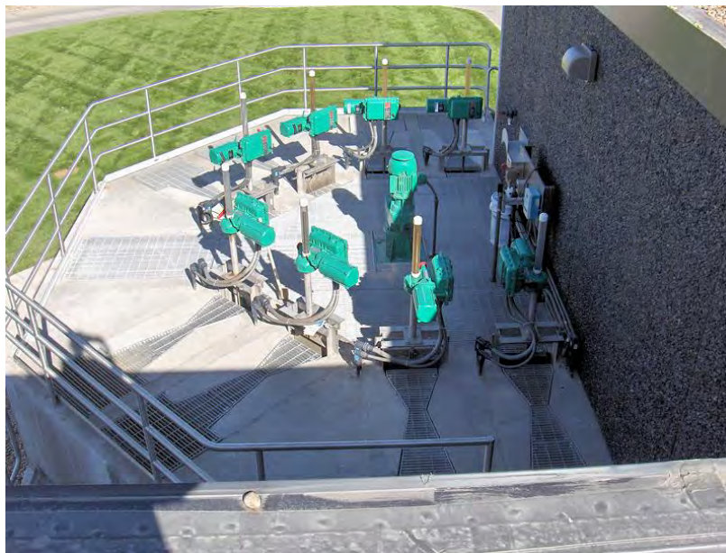
Fig 1. WAS Splitter Box
