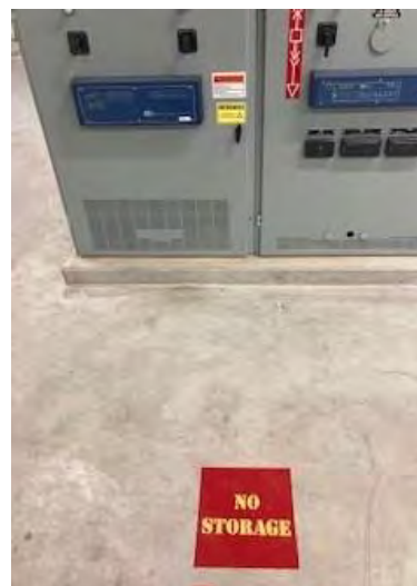
New “No Storage” signage
