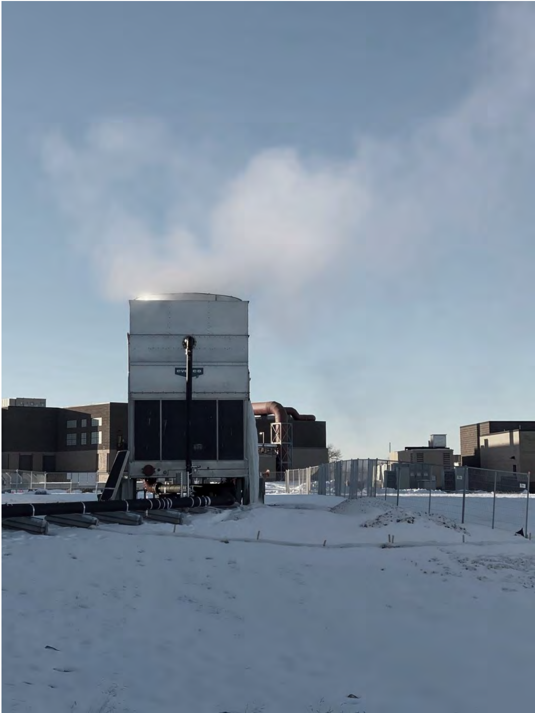
Cooling Tower in Operation
