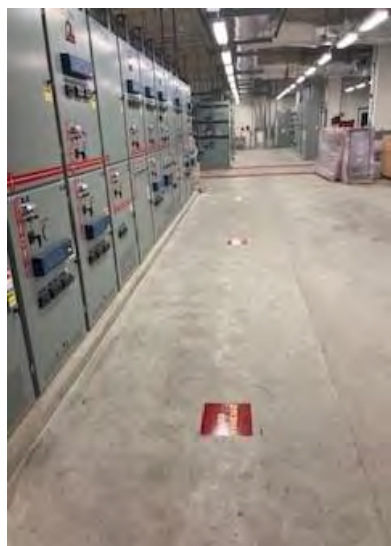
New signage provides clearance around electrical equipment
