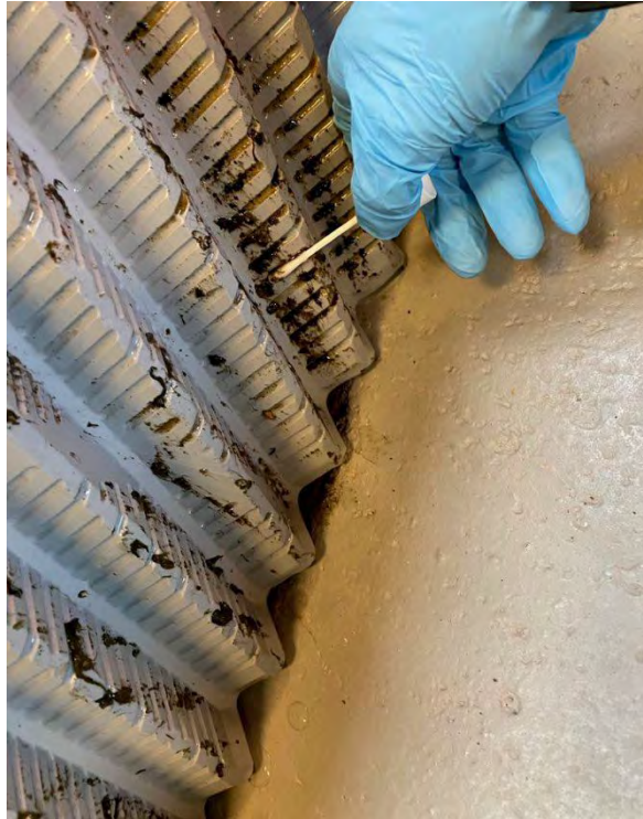
Cooling Tower Icing and Growth
