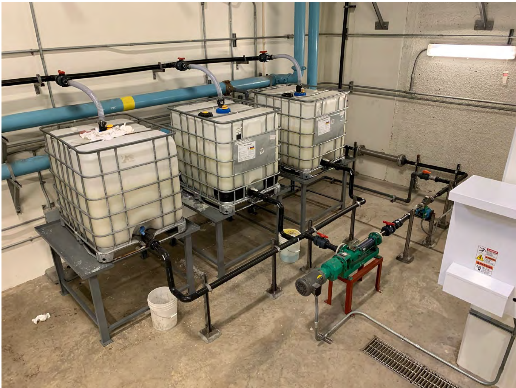
Polymer Dosing System in West RAS Pump Station (SSEC)
