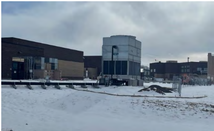
NTP's demonstration Cooling Tower.
