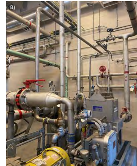
Safety improvements to the 910 Cogeneration facility which improves gas conditioning reliability and eliminates potential methane releases.
