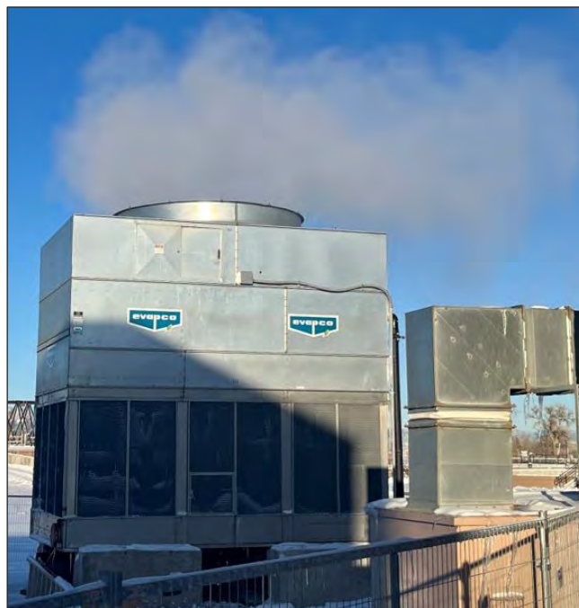
NTP effluent temperature demonstration cooling tower
