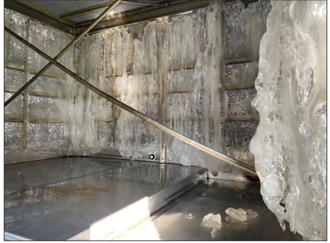
Ice inside the cooling tower (formed at 28.4°F)
