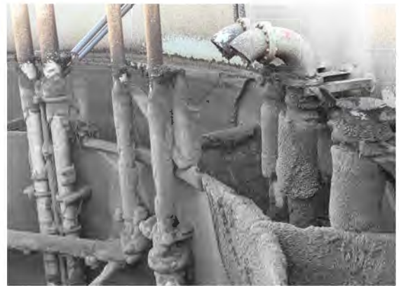
Struvite accumulation in top of reactor.
