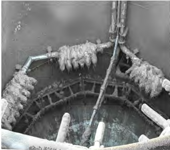
Struvite buildup in reactor.
